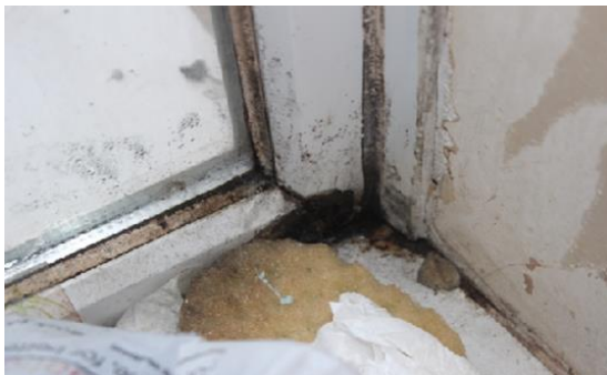
Damp on walls, ceiling and windows in all three Bedrooms
